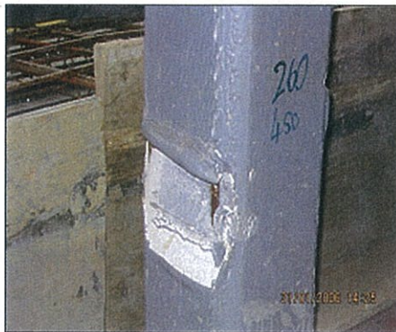
(b) Damage to coating on site
