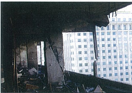
Fig. 21: Shear failure of a concrete column following a fire (due to thermal expansion)
