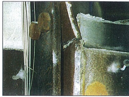
Fig. 22: Fracture of end-plate
