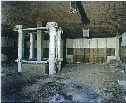
Fig. 20: Extent of spalling on the Cardington concrete fire test
